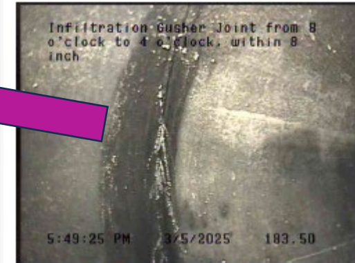
72077_352025 54926 PM.jpg, 00:16:10, 183.50ft Infiltration Runner Joint from 8 o'clock to 1 o'clock, within 8 inch
