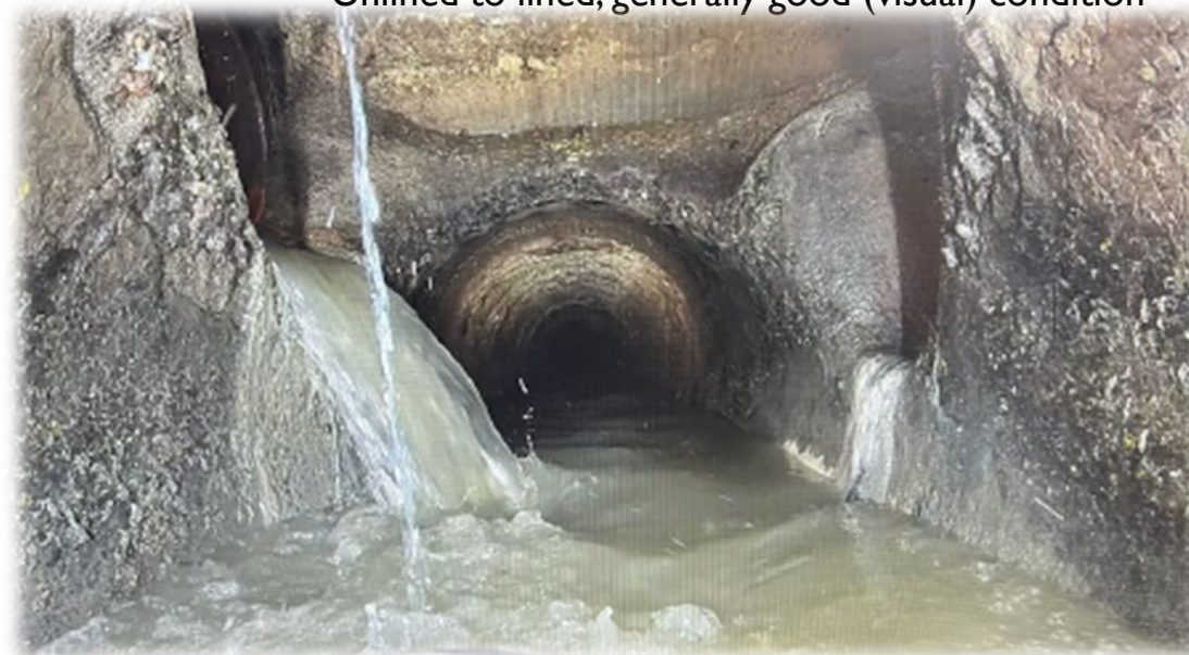
Turbulence at junctions, visible corrosion
