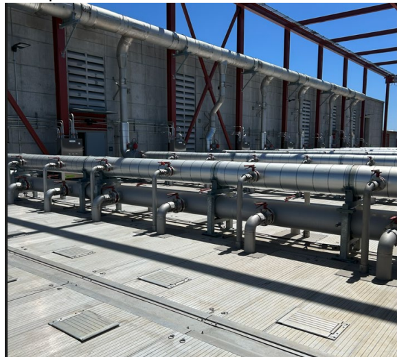
Air Piping for MLE/MBR Process
