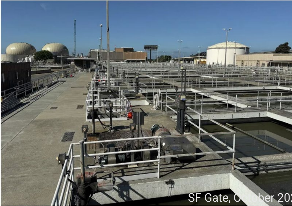
The East Bay Municipal Utility District wastewater treatment plant in Oakland, Calif., processes an average of 50 million gallons of raw sewage per day. Courtesy of Liam O'Donoghue
