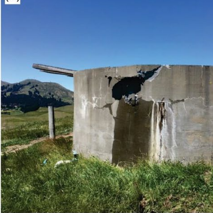
Figure 6. Ferrocement tanks at Ward, installation has collapsed (Photo: Marlborough District Council).
