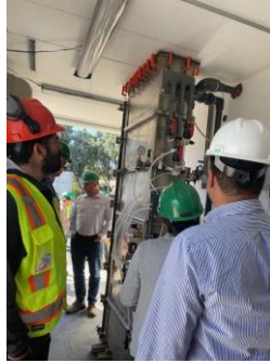
Pilot test of MABR at Central San
