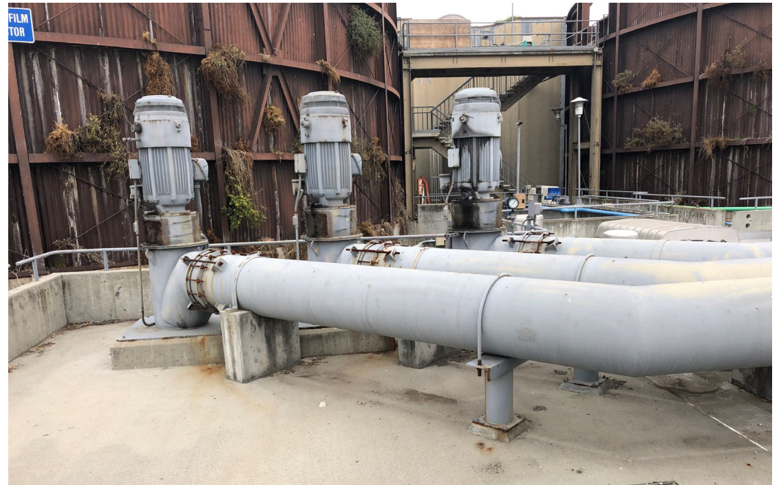
Fixed Film Reactors (1980) Intermediate Lift Pumps (1988)
