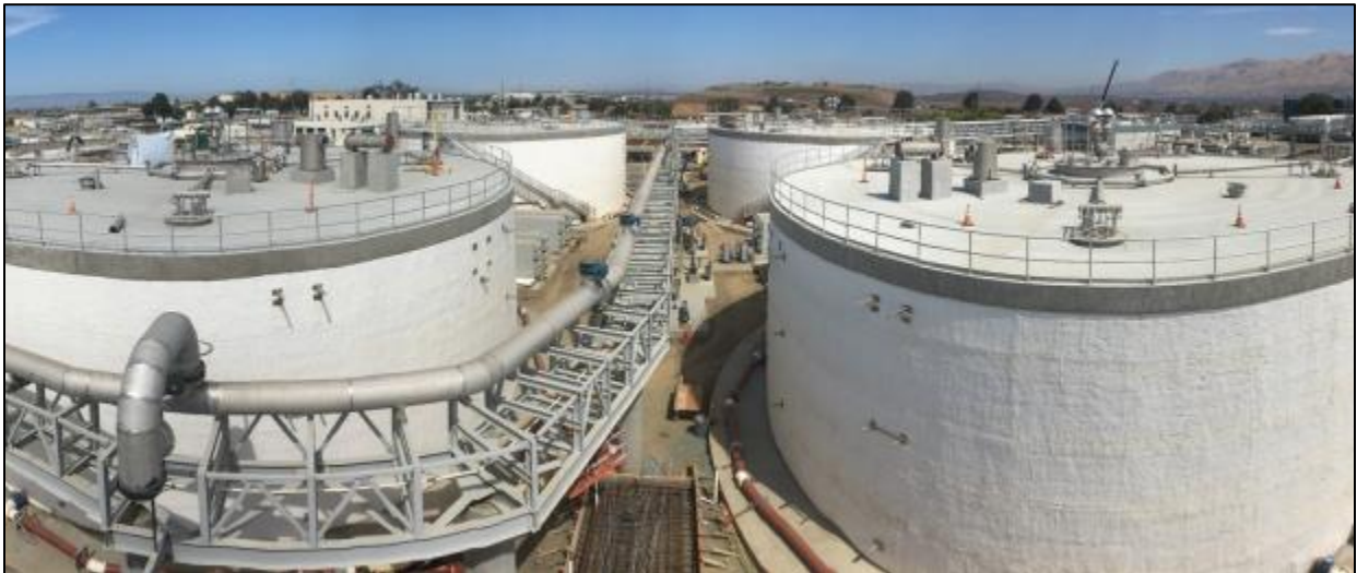
Photo: Upgraded Digesters for Temperature Phased Anaerobic Digestion at San José-Santa Clara Treatment Plant. Source: City of San José .
