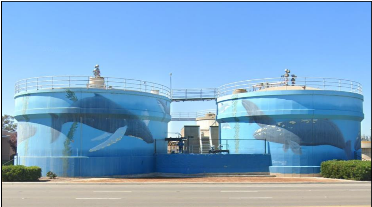
Photo: Anaerobic Digesters at City of Livermore Water Reclamation Plant. Source: Google Maps.
