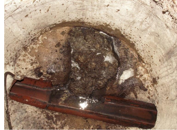
Avoided Sanitary Sewer Overflow (SSO)
