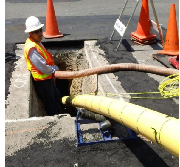
New main installation
