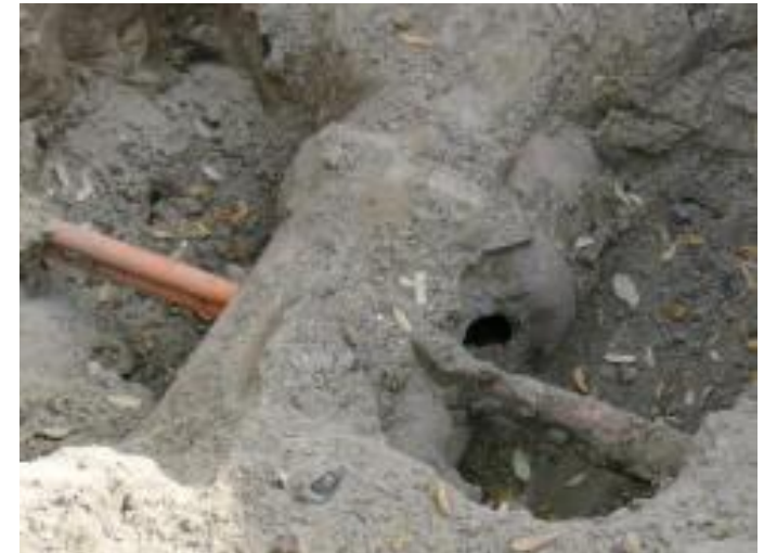
Gas Cross Bore
