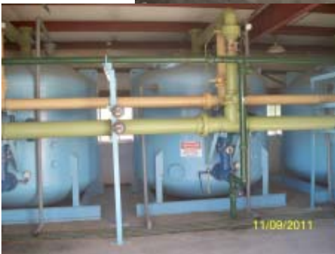
Green Sand Filter Tanks
