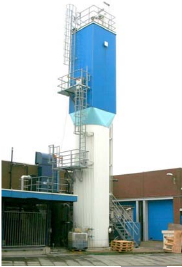
Figure 6. Anammox Reactor at Rotterdam WWTO, NL
