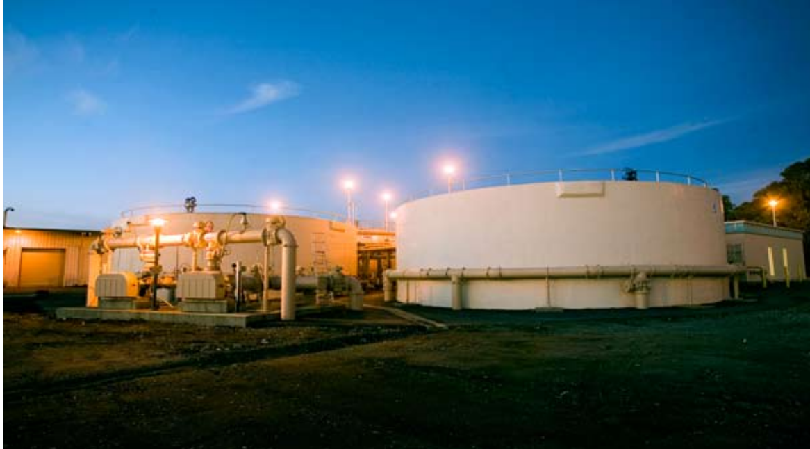
Treatment tanks at Oro Loma Sanitary District, San Lorenzo
