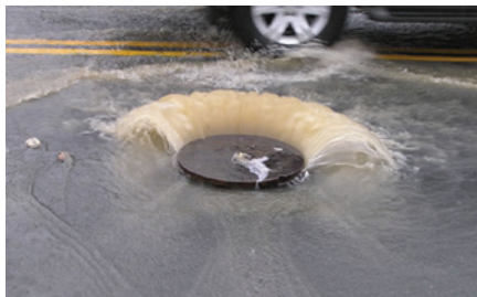
Wastewater agencies in the Bay Area are spending millions of dollars each year to prevent sanitary sewer overflows.
