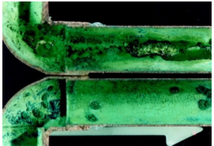
Pitting in 6-year-old cold water pipe caused by excess flux at solder joint. (2)
