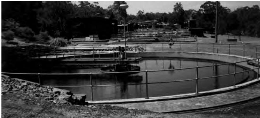
Figure 3.2. Secondary clarifier, Castle Hill STP
