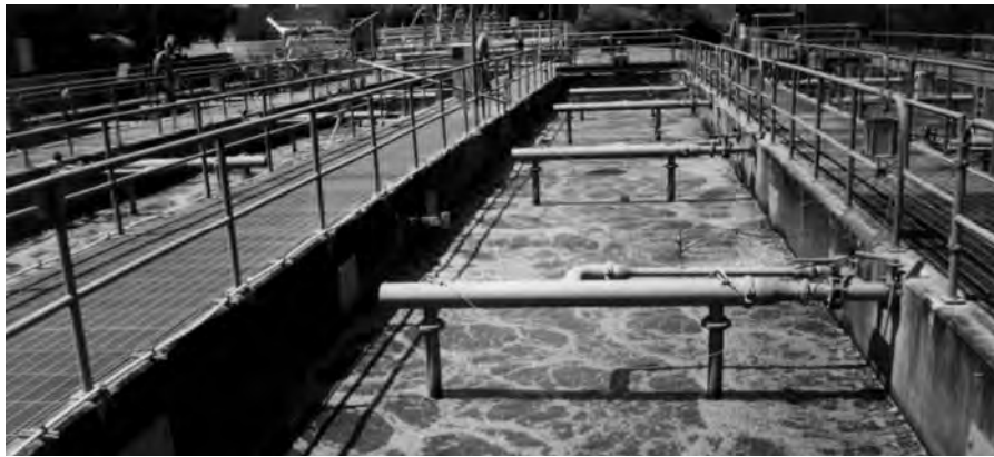
Figure 3.1. Aerated activated sludge treatment tanks, Castle Hill STP
