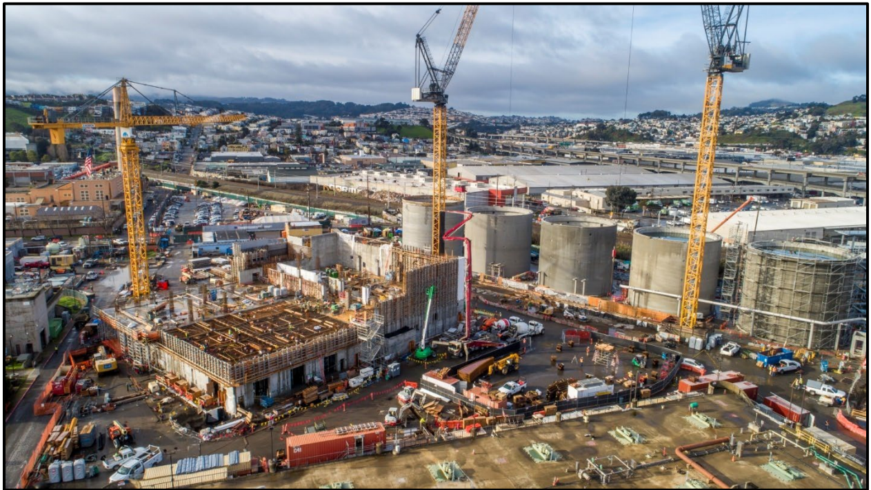
Photo: Biosolids Digester Facilities Project construction underway at SFPUC's Southeast Treatment Plant. Source: SFPUC .
